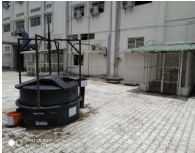
Bio Gas plant
