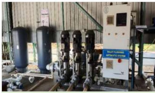
Toilet Flushing Automatic System
