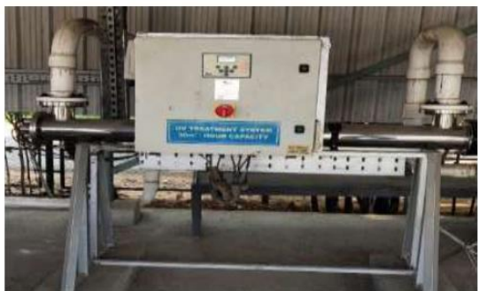
UV Treatment System
