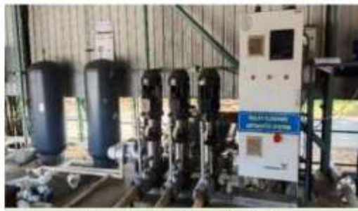
Toilet Flushing Automatic System
